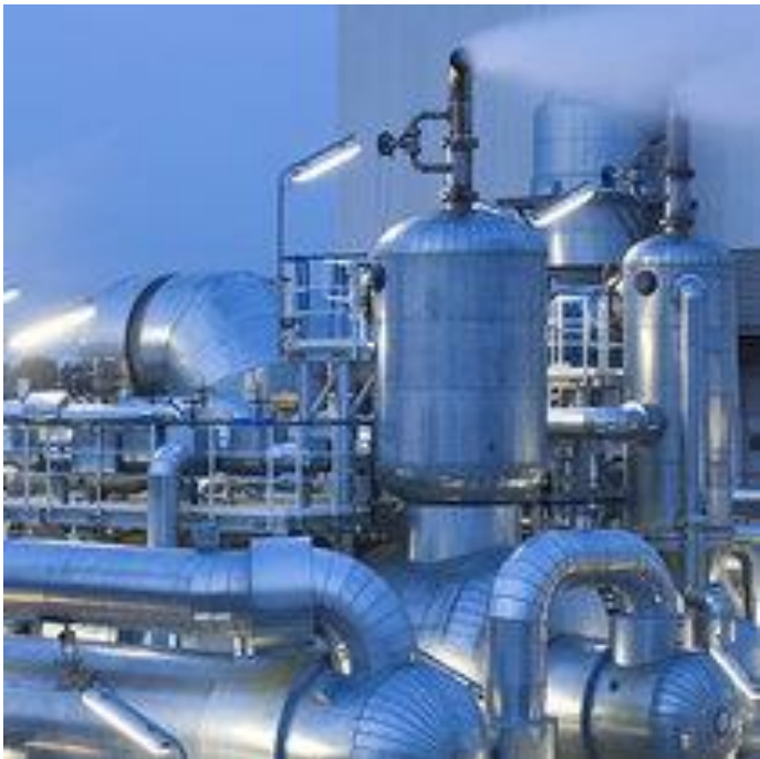
Steam methane reforming Source: Air Liquide
