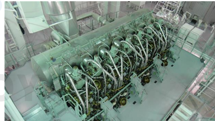
MAN B&W ME-LGI Engine and Fuel Supply System
